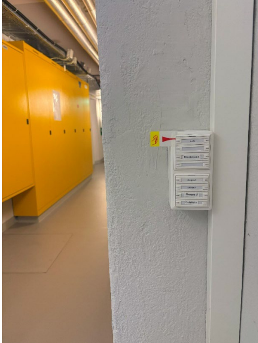
Corridor switch panel
